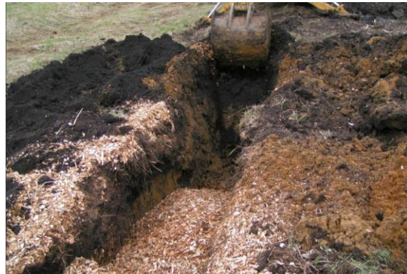
Construction of trench for woodchip bioreactor. Photograph from presentation "Anaerobic Woodchip Bioreactors Under Minnesota Conditions," courtesy of Andry Ranaivoson, University of Minnesota
