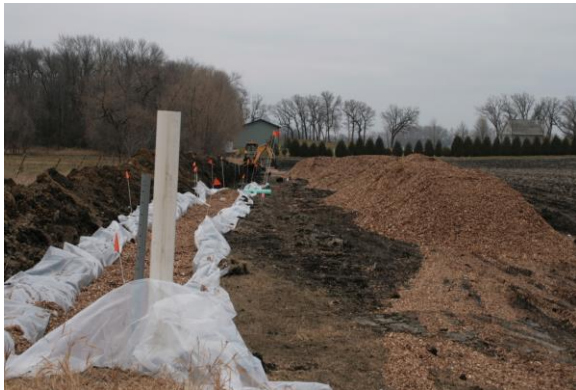
Construction of woodchip bioreactor. Photograph from presentation "Anaerobic Woodchip Bioreactors Under Minnesota Conditions," courtesy of Andry Ranaivoson, University of Minnesota
