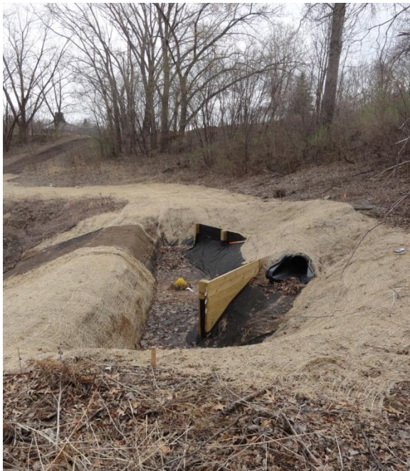
Spent-lime treatment system upstream of Wakefield Pond during construction before spent lime has been added.
