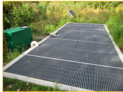
Figure 4-30 Spent Lime Treatment System
