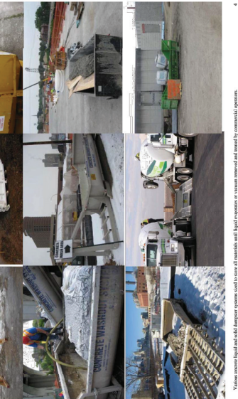
Yellow concrete liquid and solid separator system used to store all materials until liquid separator or system removed and used by commercial operators.
