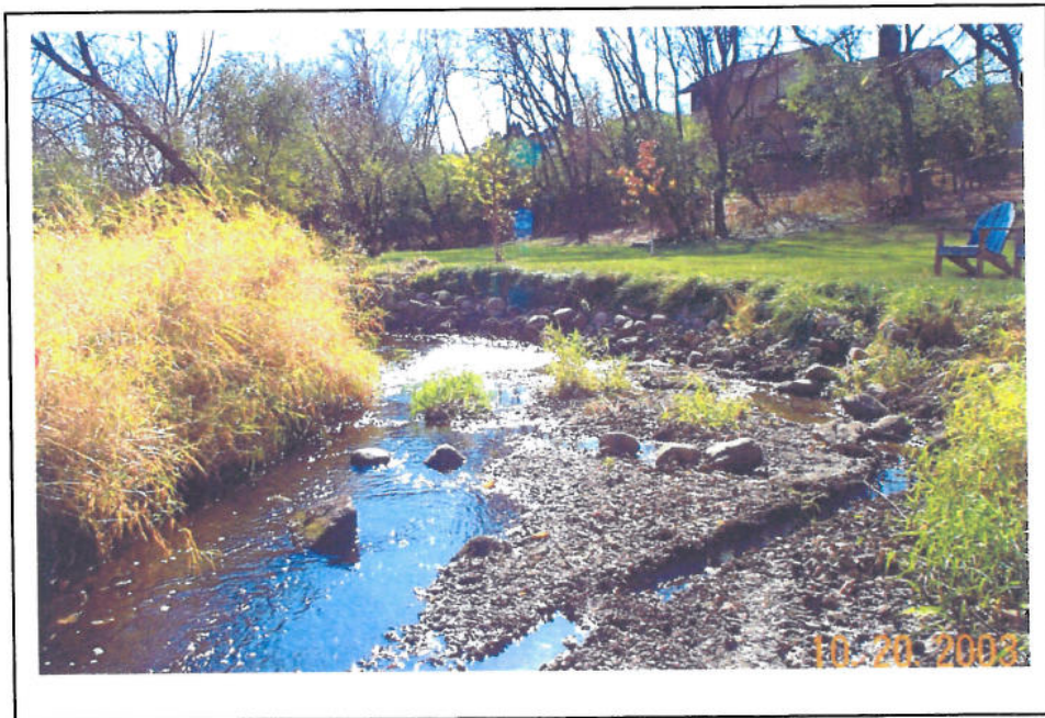
Figure PC25 – Reach P-6 Erosion at Turf Yard
