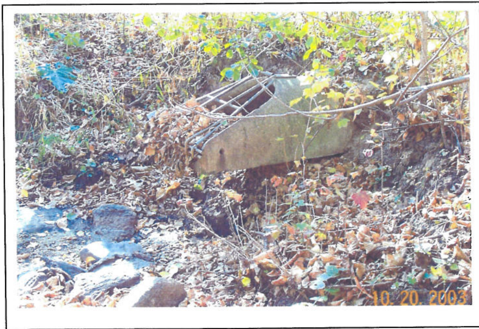
Figure PC28 - Reach P-7, Significant Downcutting at Pipe Inlet
