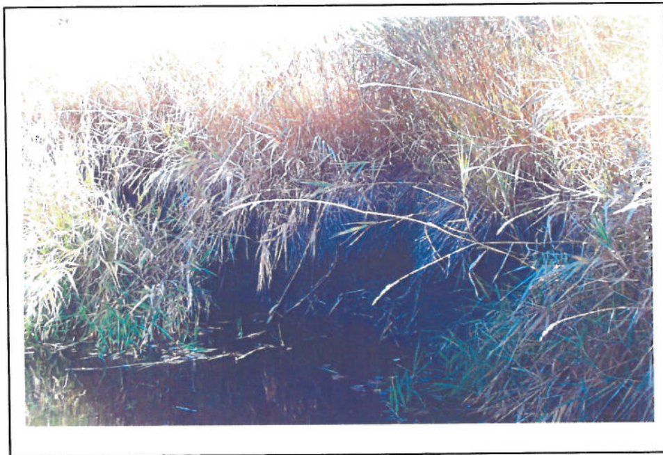
Figure PC13 - Reach P-2 Bank Erosion
