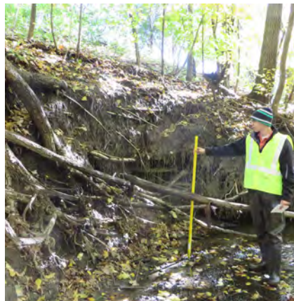
An eroded bank on Riley Creek that might benefit from stabilization.
