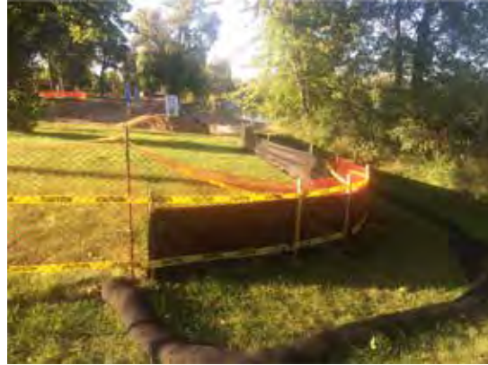
Temporary and permanent erosion control measures are essential to reducing pollution in runoff
