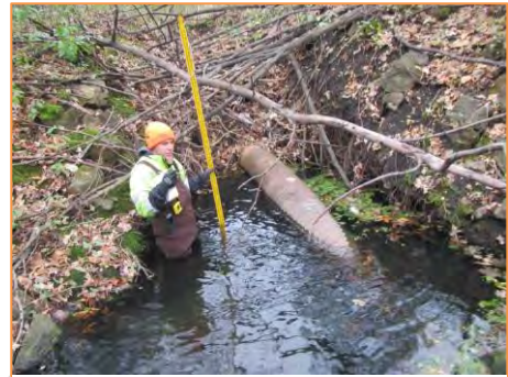
Figure 4.4-1 Degraded Stormwater Culvert PT2B
