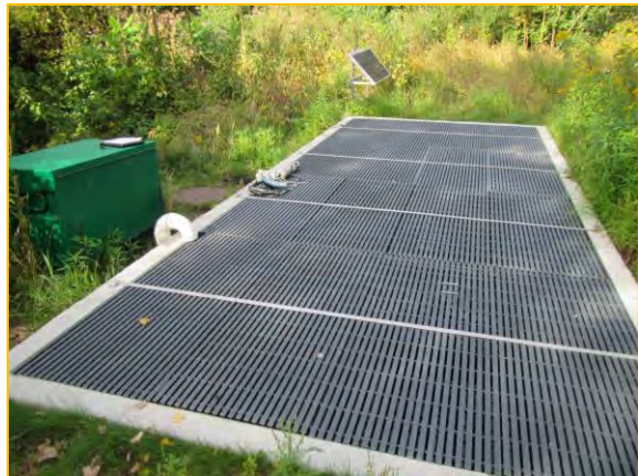
Figure 4.9-1 Spent Lime Treatment System
