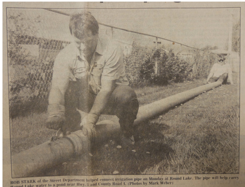
Setting up an emergency water pump (EPN)
