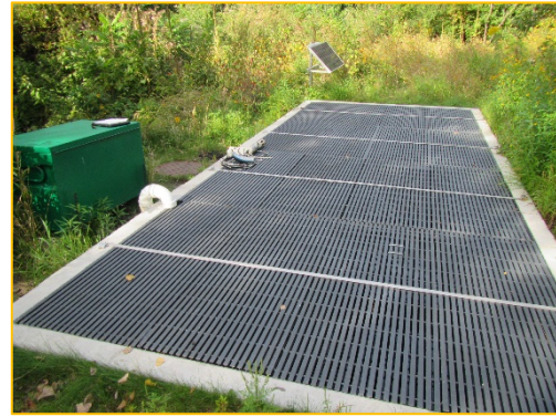
Figure 4-28 Spent Lime Treatment System
