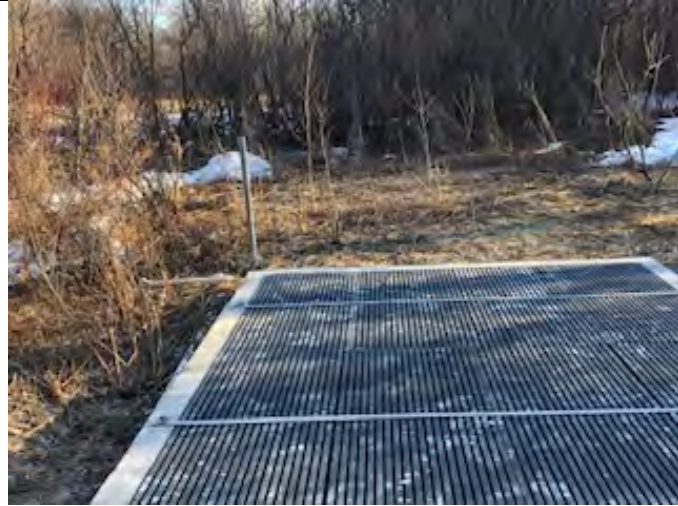
Photograph 1. Photograph taken on March 13, 2020. The contractor has substantially completed modifications to the system. Final site restoration will occur later this spring.
