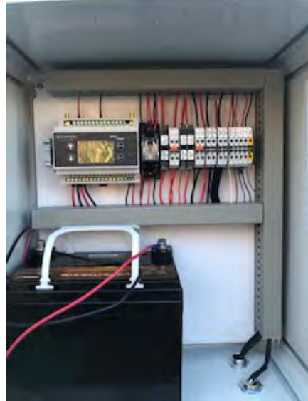
Photograph 2. Photograph taken on March 13, 2020. The inside of the control box for the automated water level control structure. The control box and solar panel are located on a pole adjacent to the filtration system. Staff will be programming the automated water level control structure this spring and will bring the system online after verification that the water level control structure is operational.
