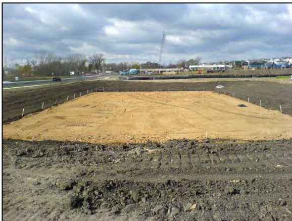
Construction of Beam Avenue iron-enhanced sand filtration system (Ramsey-Washington Metro Watershed District, 2017).
