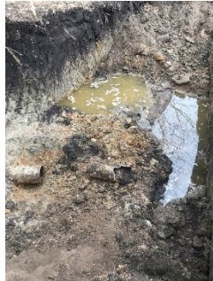
Excavated forebay and exposed existing drain tile to tie into to level control structure
