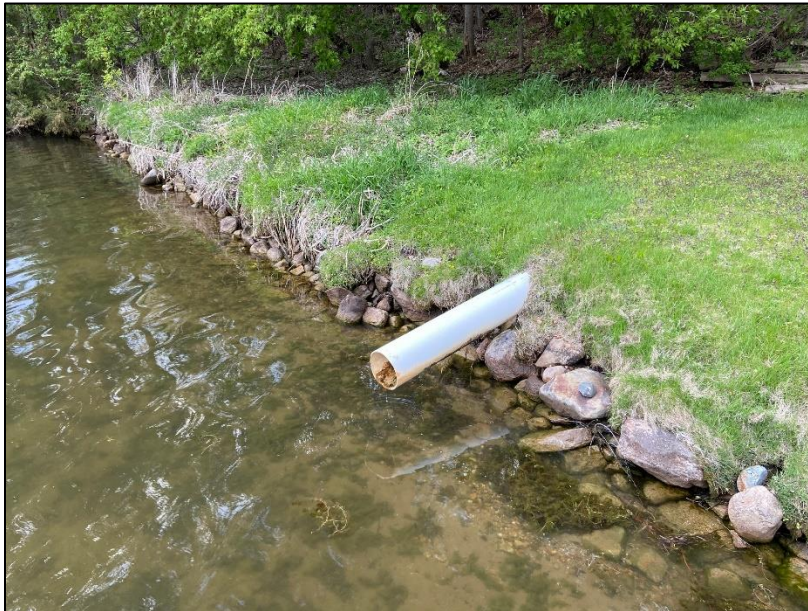
Figure 3. Pipe Protruding from Bank on Neighboring Property
