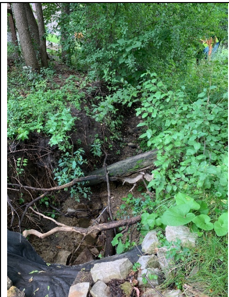
Photo B of existing severe erosion at Site 5
