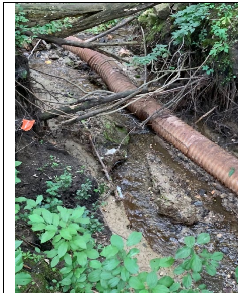
Photo A of existing outlet pipe and severe erosion at Site 4
