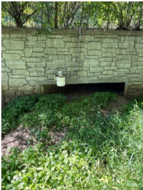
Sediment delta on downstream end of north culvert
