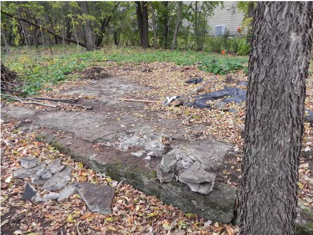
Historic foundation with concrete slab within. We want to remove the slab.
