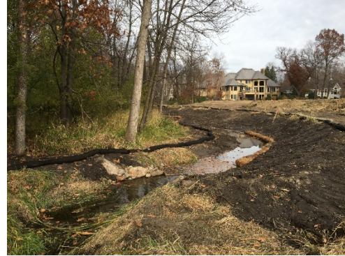
North site – looking northerly at boulder vane, coir log, and new creek alignment - November 8, 2021
