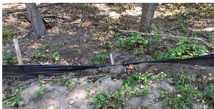
District staff inspect project sites and direct permit holders to take corrective actions as needed to protect water quality. The image above shows a silt fence violation (failure) at a site in 2022.
