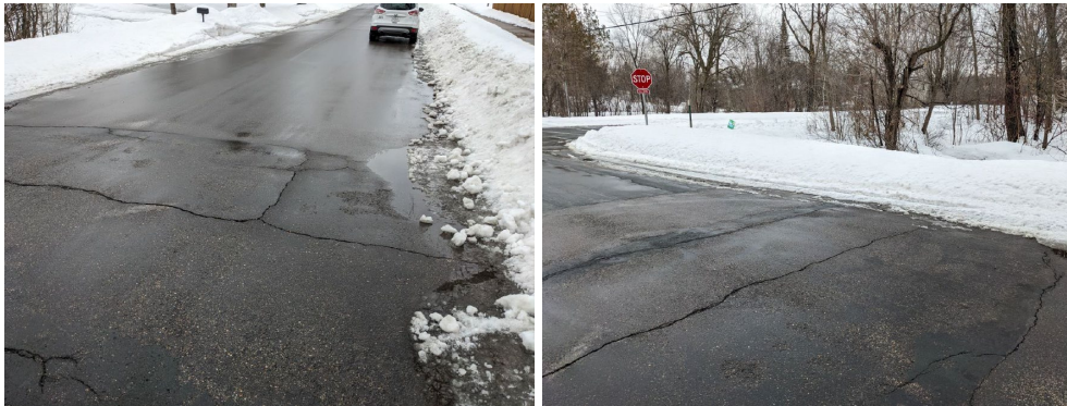
Photos of heaving pavement over culvert crossing
