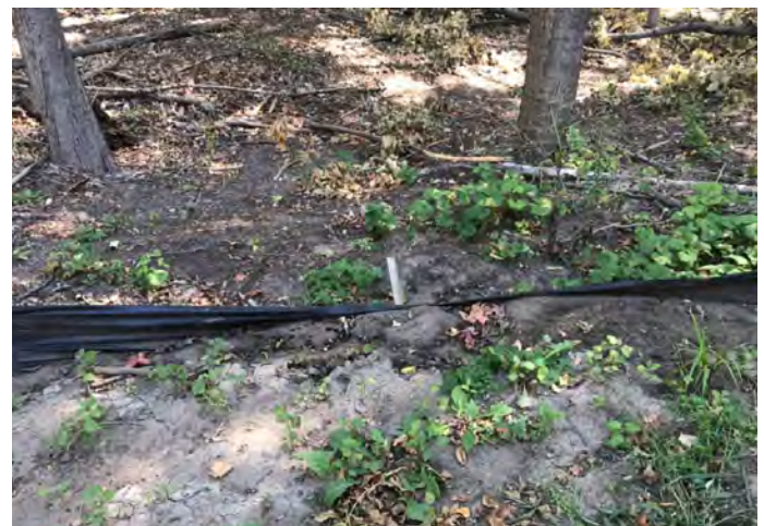
District staff inspect project sites and direct permit holders to take corrective actions as needed to protect water quality. The image above shows a silt fence violation (failure) at a site in 2022.
