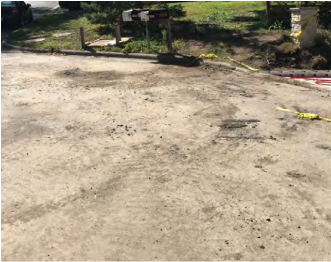
The image above shows tracking of sediment onto a street from a 2022 construction site, which violates District permit rules.
