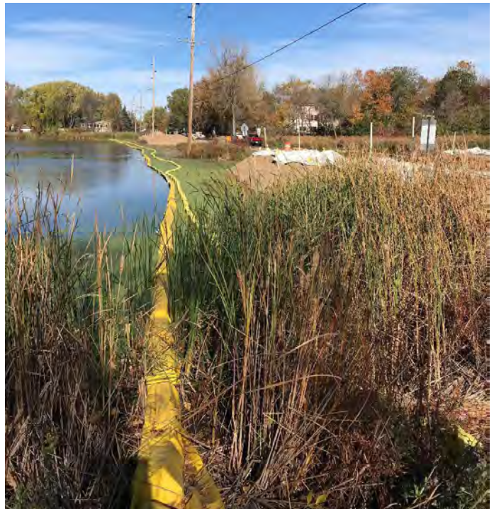
A double row of yellow silt curtains in the water protect the lake from the Duck Lake Road construction zone (fall 2021).
