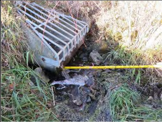
IMG-0258 Stormwater culvert along right bank, undercut 0.6m
