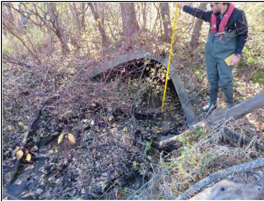
IMG-0204 Facing upstream, culvert under Park Drive, culvert 40% filled
