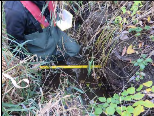
IMG-0209 Bank undercut on both sides by about 0.4m
