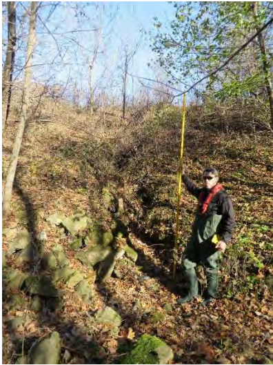
IMG-0185 Drainage from road causing small ravine erosion
