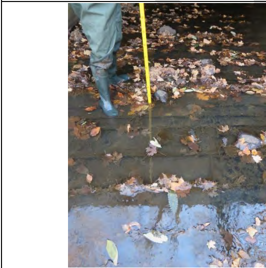
IMG-0237 Exposed rebar inside culvert
