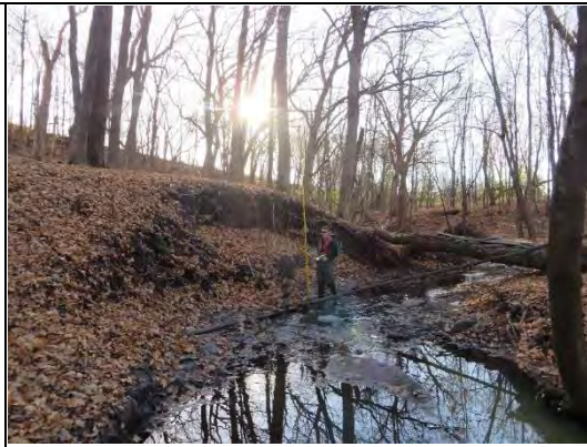
IMG-0232 Erosion on left bank measuring 2.7m by 6m wide; downed tree with wood plank bridge
