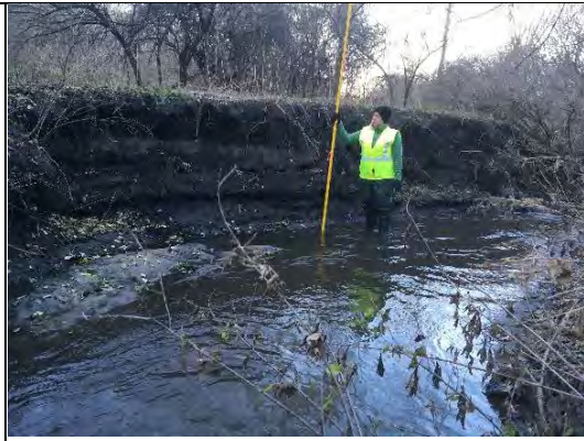
IMG-0325 Erosion 1.5m by 5m long; sand/silt deposition
