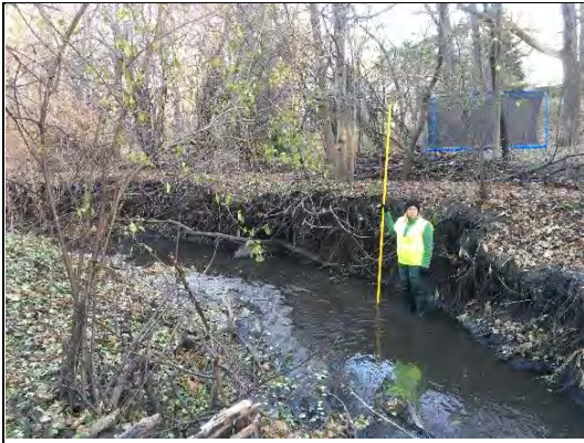
IMG-0324 Erosion on right bank measuring 1.6m by 6m long
