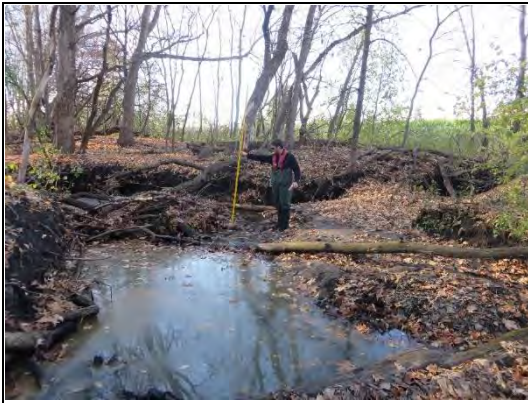
IMG-0231 Large woody debris dam
