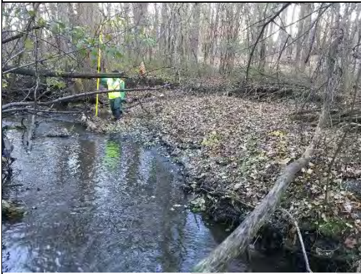
IMG-0328 Signs of major bank sloughing, partially healed over; right bank
