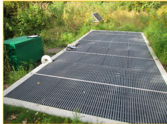
Figure 34 Spent Lime Treatment System
