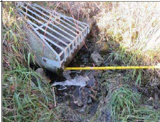
IMG-0258 Stormwater culvert along right bank, undercut 0.6m
