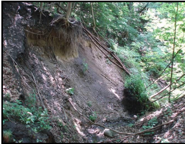
Figure 4.24 Severe erosion in upper part of main ravine (Site 12)
