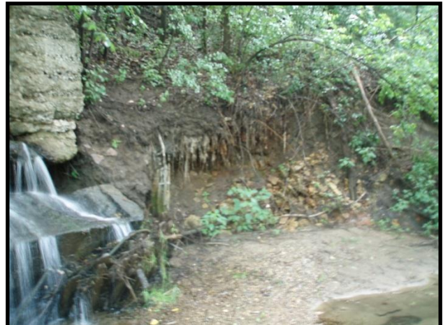
Figure 4.3 Large bank failure downstream of culvert outlet on left bank (Site 1)
