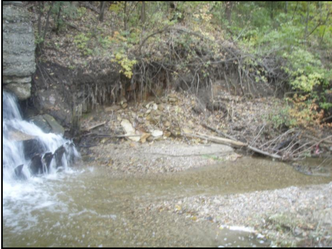
Figure 3.2 Eroding left stream bank immediately downstream of culvert outlet
