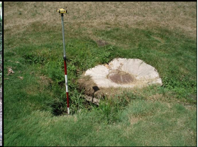
Figure 4.9 Pipe inlet in poor condition from east end of golf course parking lot (Site 4)
