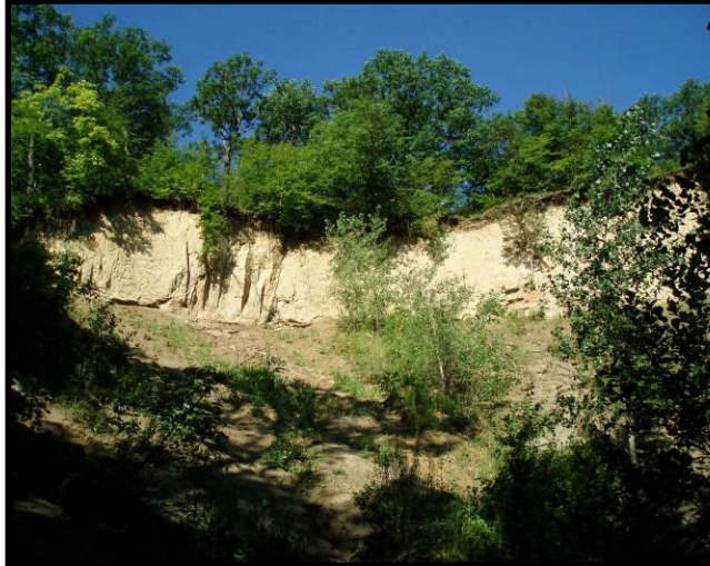
Figure 4.28 Large slope failure with wet soils on lower area and dense sandy clay soils on upper bank (Site 14)
