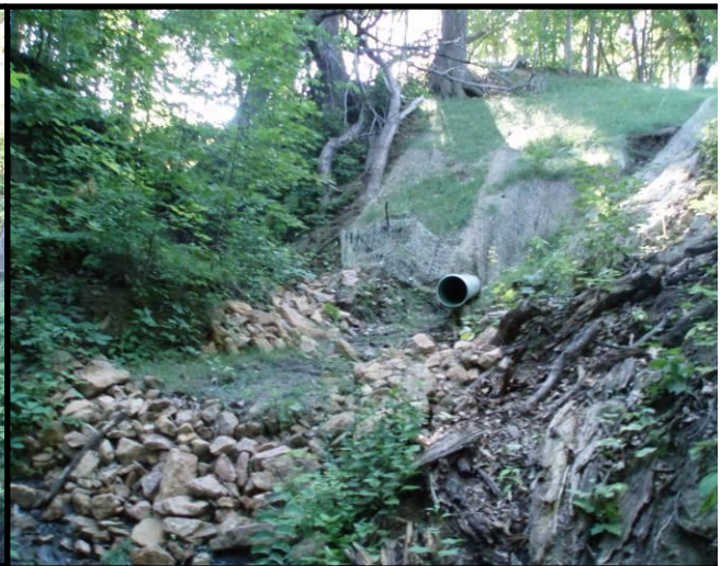
Figure 4.31 New pipe outlet from golf course (Site 15)
