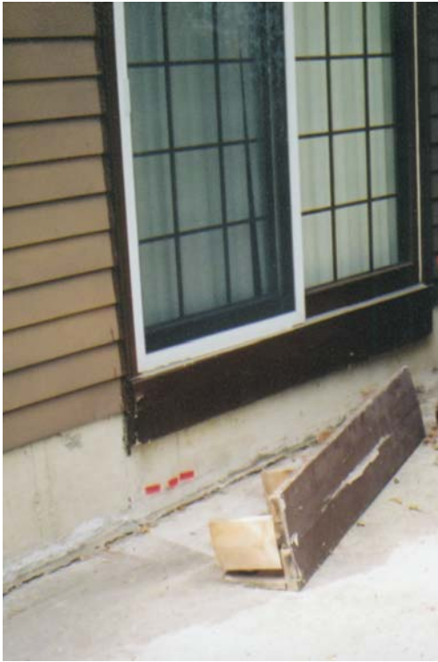
Figure 5.5: A home damaged by soil settling.
