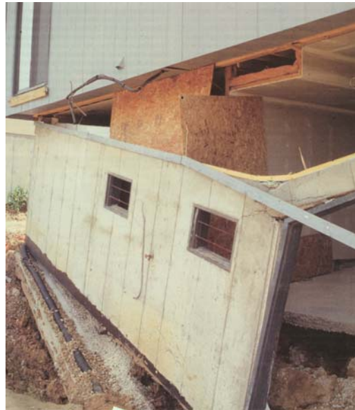
Figure 3.7: A home damaged by slippage of shale beds.
