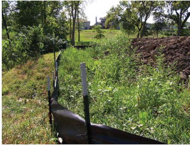
Figure 3.10: Silt fences collect sediment and keep it from reaching water bodies near construction sites. Construction is just starting on this site.
