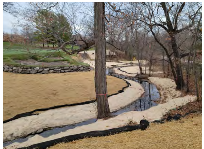
Re-meandering and bank stabilization of Riley Creek within Bearpath Golf and Country Club in November 2021.
