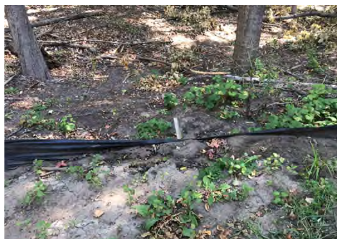
District staff inspect project sites and direct permit holders to take corrective actions as needed to protect water quality. The image above shows a silt fence violation (failure) at a site in 2022.
